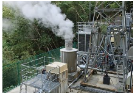
Binary cycle power generation (Shimoda Hot Springs)
