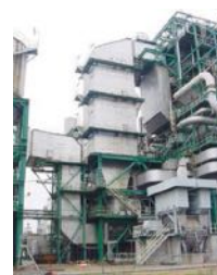
Flue gas denitrizer
