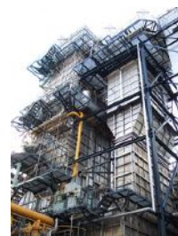
Flue gas desulfurizer
