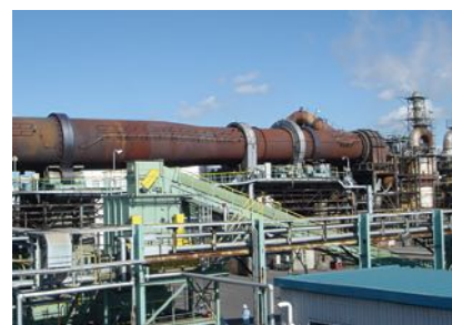
JX Metals Tomakomai Chemical rotary kiln furnace
